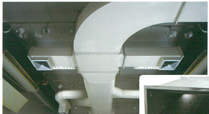
Internal Ducting Systems
